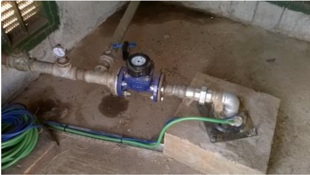
Figure 6.10 One of the communal boreholes to supply water for Mbaula.
