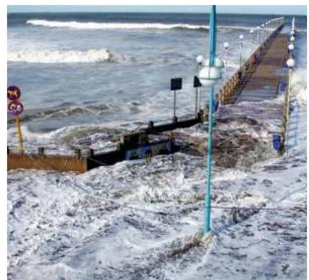
Damage from the March 2007 storm in KwaZulu Natal by high sea-levels and large waves; Top: Beach facilities on the lower South Coast; Middle: Flooding of George Hulett Place, Salt Rock; Bottom: Inundation of North Beach Pier, Durban
