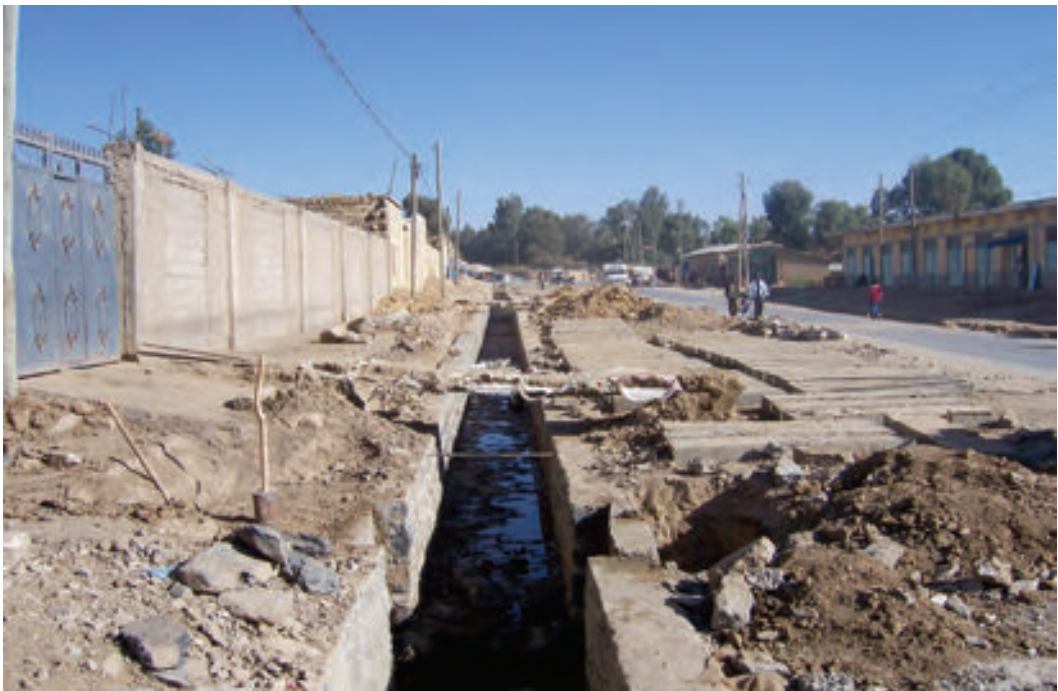
Figure 9. Substandard storm water drainage in Adigrat City (2009)
