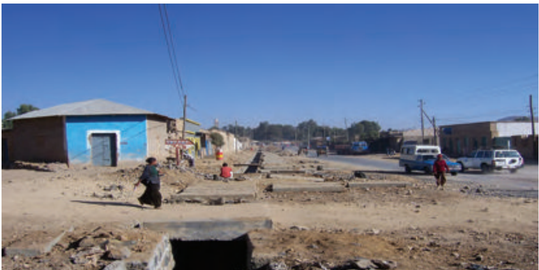
Figure 5. Poor water drainage canal in Adigrat City (2009)
