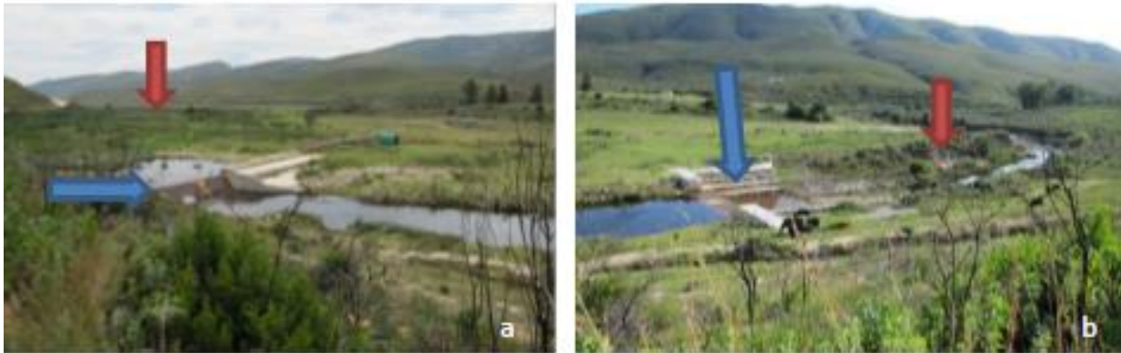
Figure 4.8: Gabion placed to protect the wetland upstream. On Figure 4.8a the gabion is shown downstream to upstream. Here the protected wetland is shown, protected by the gabion. On 4.8b the gabion is shown upstream to downstream and a lot of erosion is visible. The photos are taken by Alanna Rebelo, 2012.
