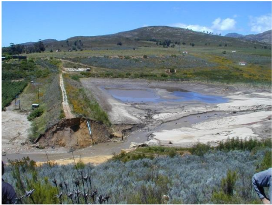
b. Dike burst after 2006 floods (2)
