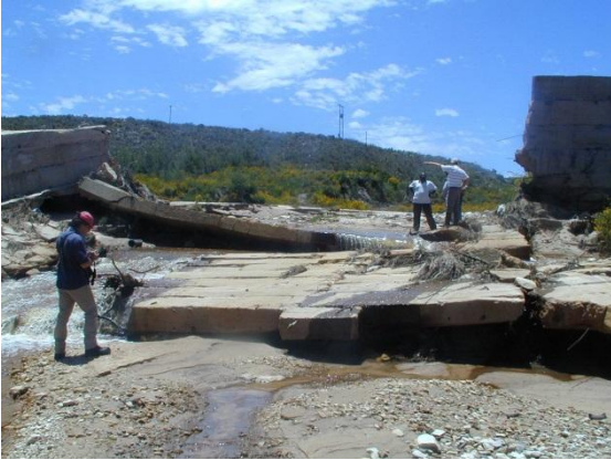
c. Damaged bridge after 2007 floods
