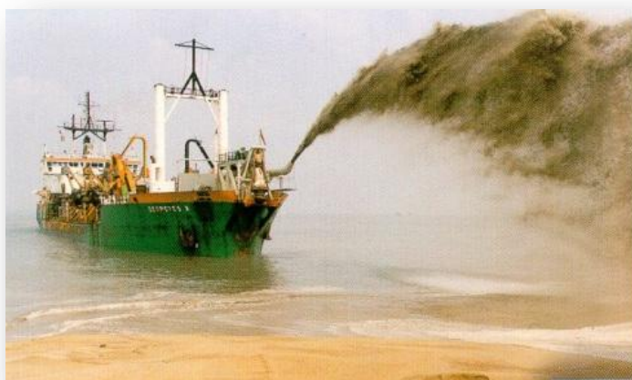
Figure 7.2: Beach nourishment by means of direct “rainbowing” of sand from the dredger to shore (only practical in certain areas).
