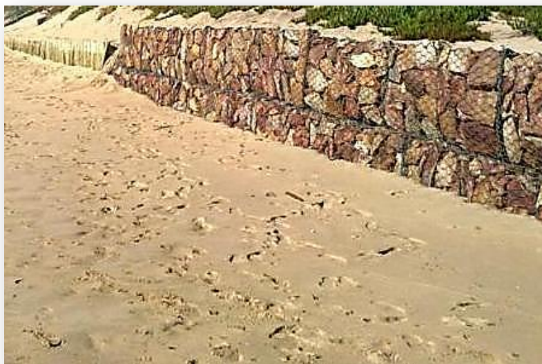
Figure 7.16: Example of a Gabion retaining wall structure (to protect the back-beach area)
