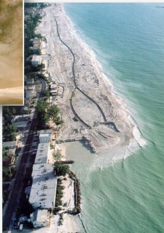
Figure 7.3: Beach nourishment by means of pumping sand onto the beach through a pipe system
